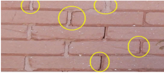
Fig.1: Cracks Formed in the Brick Mortar Joints Crack Formation Below the Load Bearing Walls
