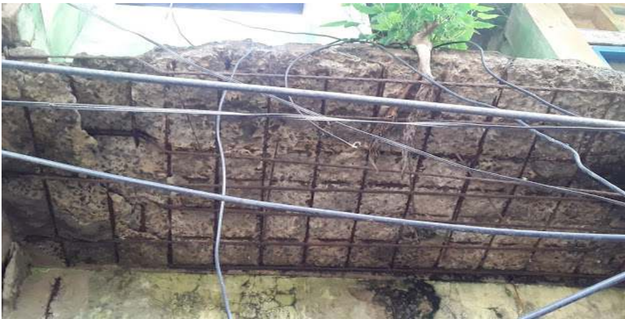
no cover block causing severe damage
