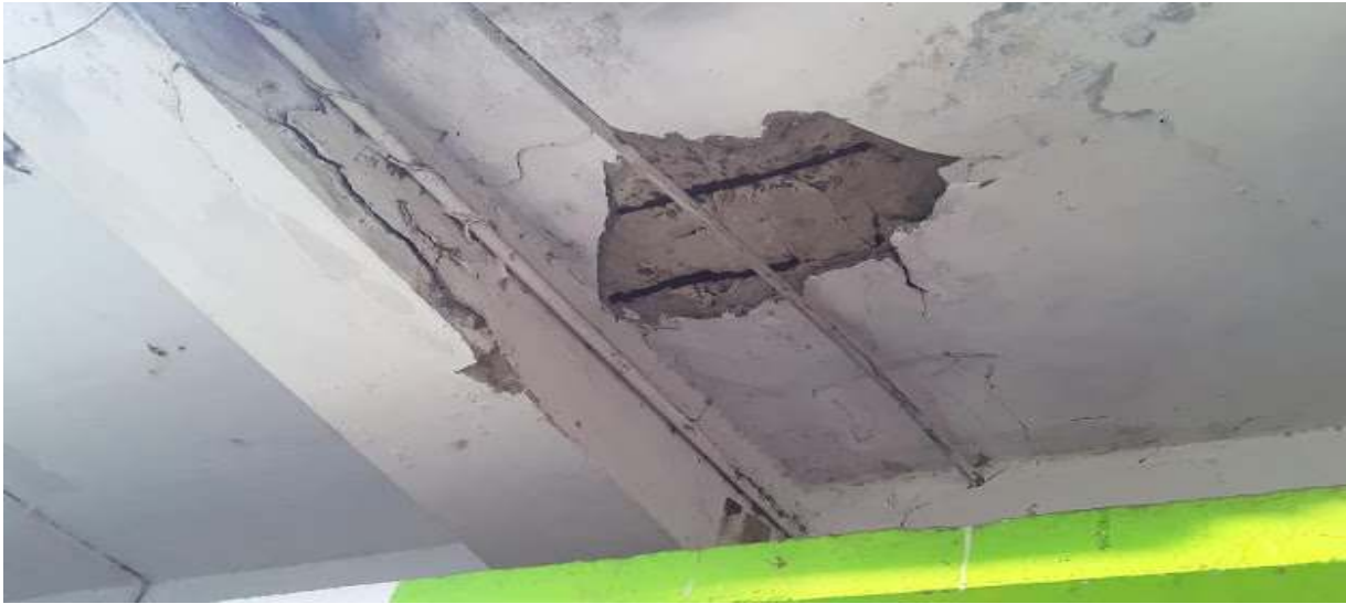
no cover block causing damage at early stage
